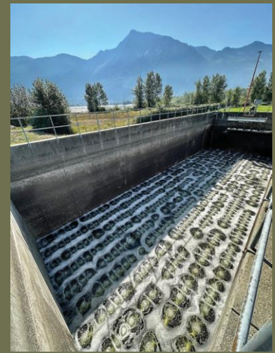
SBR #2 at the Agassiz Wastewater Treatment Plant
